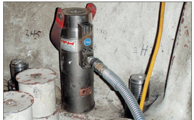
Casing bolt connection.
