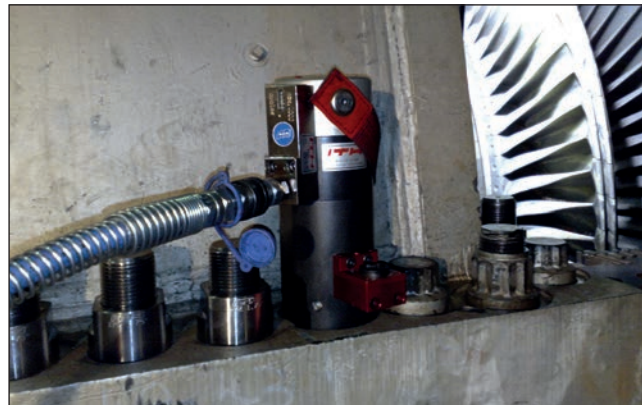
Turbine casing bolt connection.
