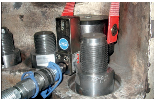
Casing bolt connection.
