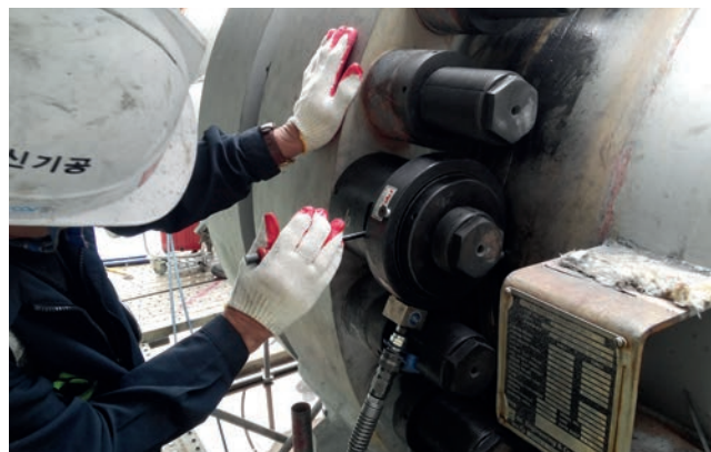
Typical ANSI flange application at a heat exchanger.
