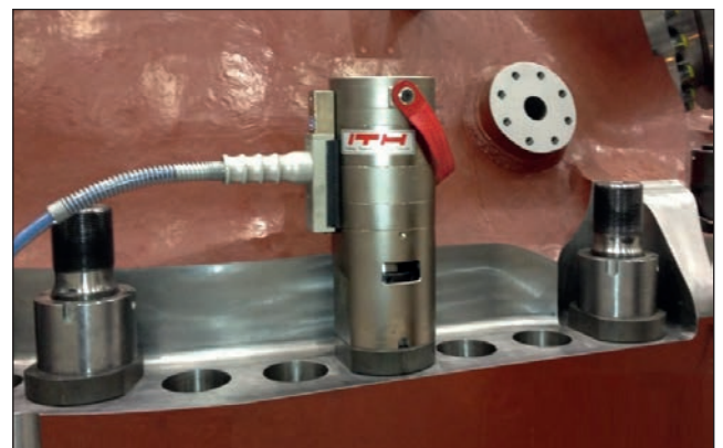
Casing bolt connection.
