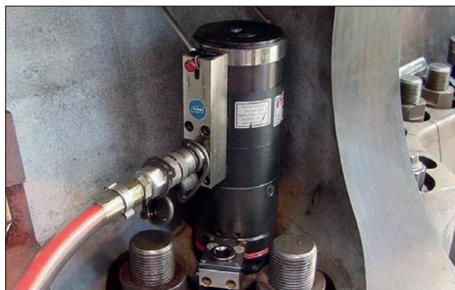
Casing bolt connection.
